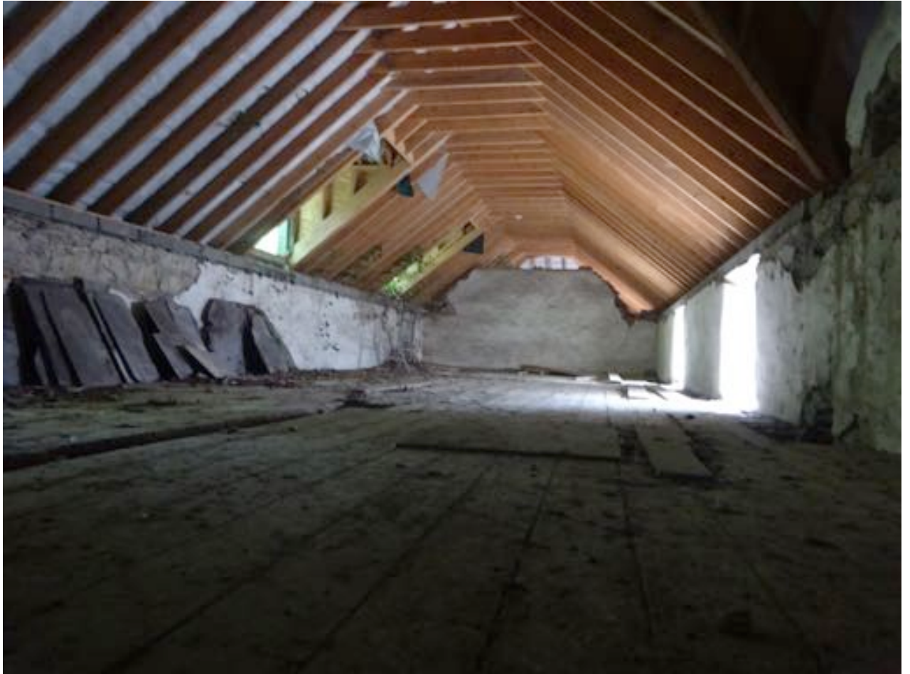
View above at first floor level (north range – Fig 70) of the stable yard buildings.
