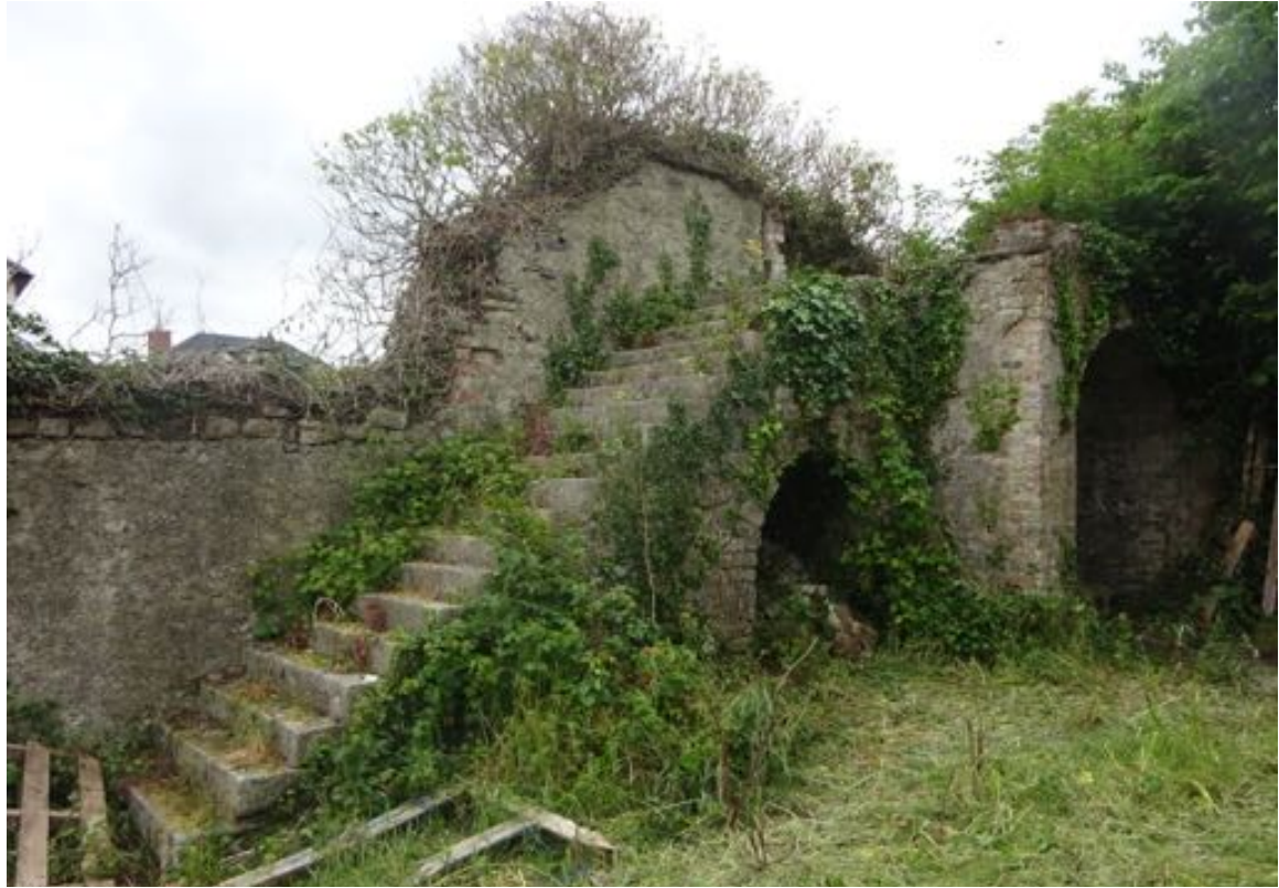
View of the more ruinous corner bastion at the south west corner of the walled garden (Fig 79).
