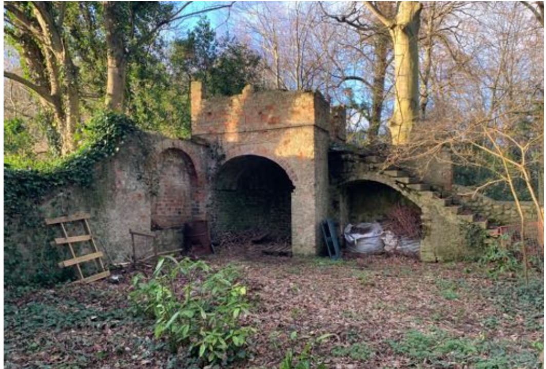
Fig 16: Internal view of the corner tower at the north western corner of the walled garden - this and the equivalent corner tower at the south west corner are to be stabilised and repaired so that they are safe and conserved as a landscape feature within the walled garden.
